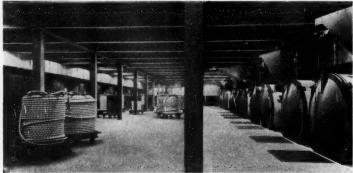
Fig. 17—Air conditioned cable storage room.
